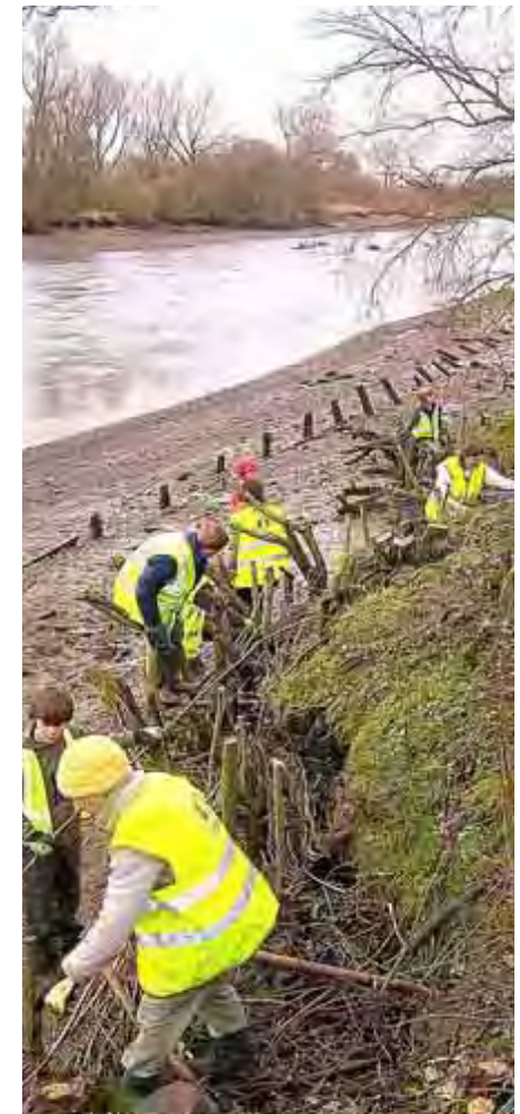
Willow spiling: a traditional conservation technique that Environment Trust volunteers have been putting into practice to protect the riverbank along Kew Reach
